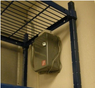
Photo 5: Defrost Time Clock
