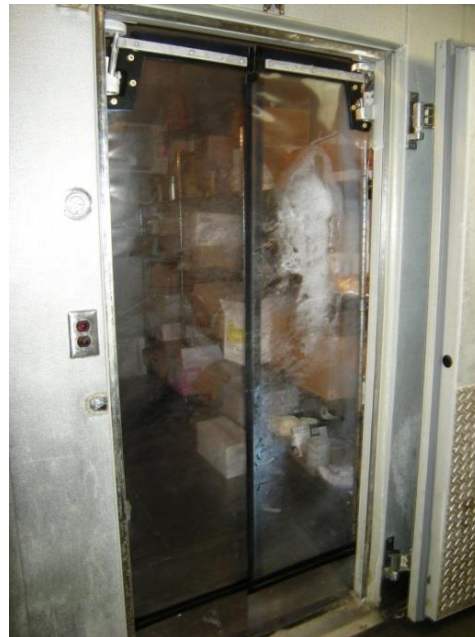
Photo 2: Walk-in Freezer with Saloon Door Curtain
