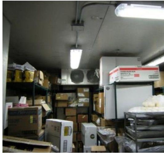
Photo 8: No Ice on Ceiling after Retrofit
