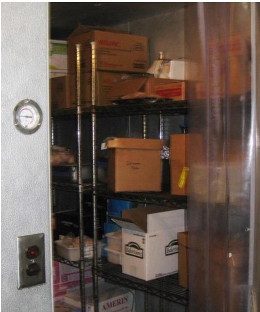
Photo 1: Walk in Freezer with Strip Curtains Partially Removed
