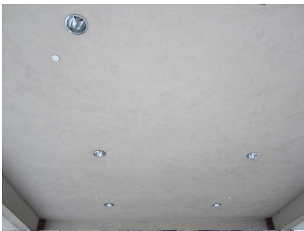
FIGURE 4: ENTRANCE CANOPY LIGHTING
