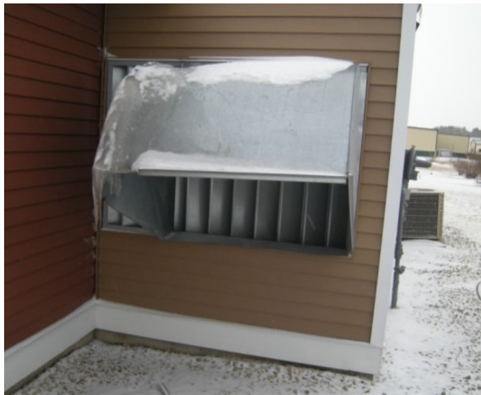
Figure 16: Outdoor Air Damper at 100%
