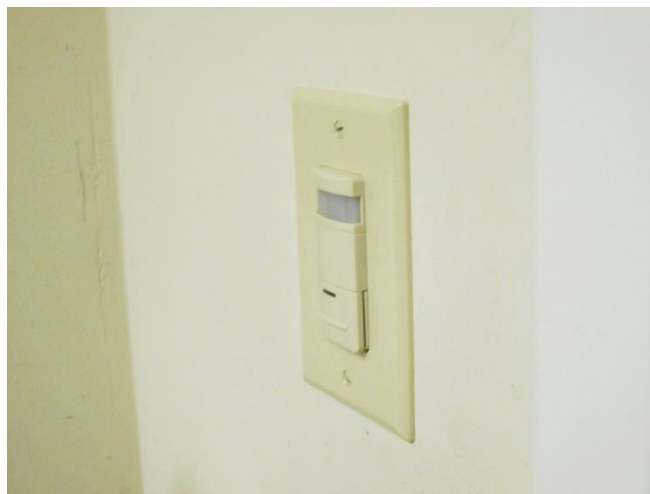
FIGURE 11: EXISTING OCCUPANCY SENSOR
