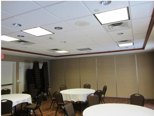
FIGURE 6: CONFERENCE ROOM LIGHTING
