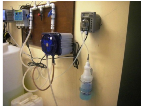
FIGURE 3: FEED SYSTEM FOR LIQUID POOL COVER
