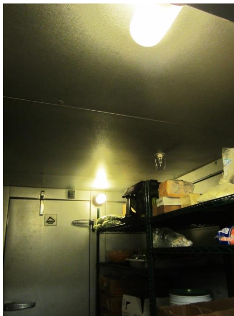
FIGURE 10: WALK-IN COOLER LIGHTING
