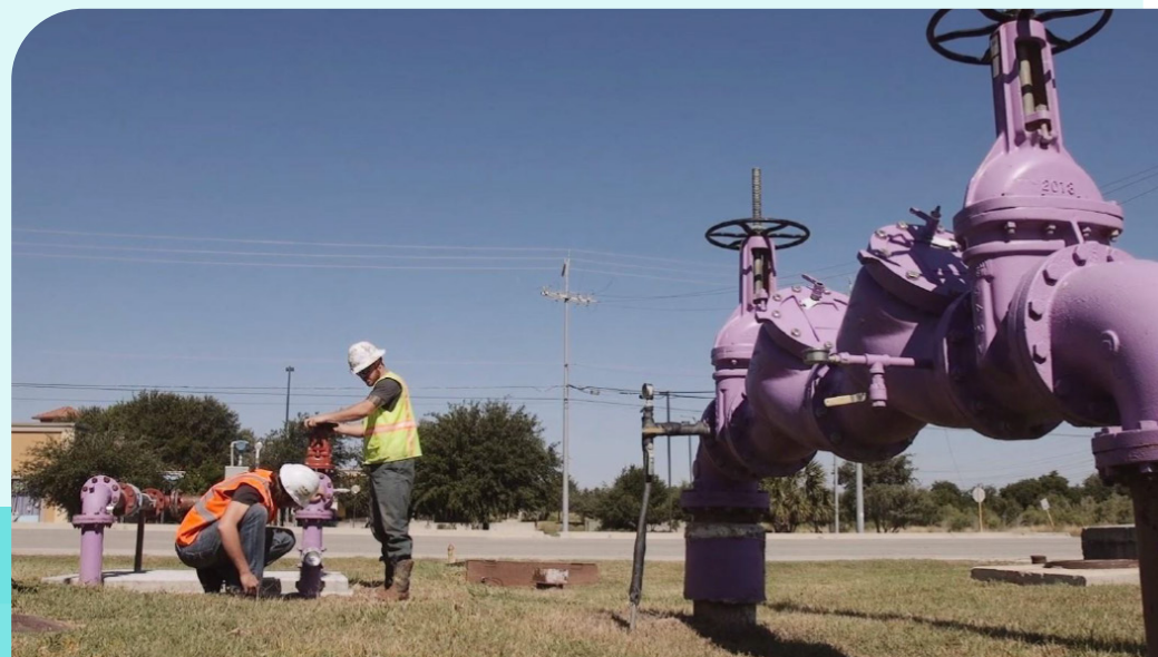
SAWS crews found and opened dozens of accidentally closed valves that had been constricting water flow in the distribution system. The change is reducing friction and saving energy. (Photo courtesy of SAWS)
