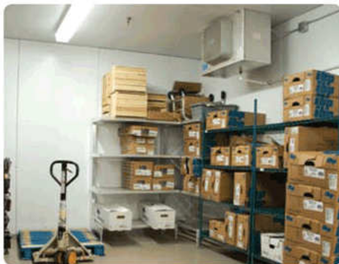
Remind customers to avoid placing items directly in front of fans, for efficient operation, and easier service access. PHOTO COURTESY US COOLER
